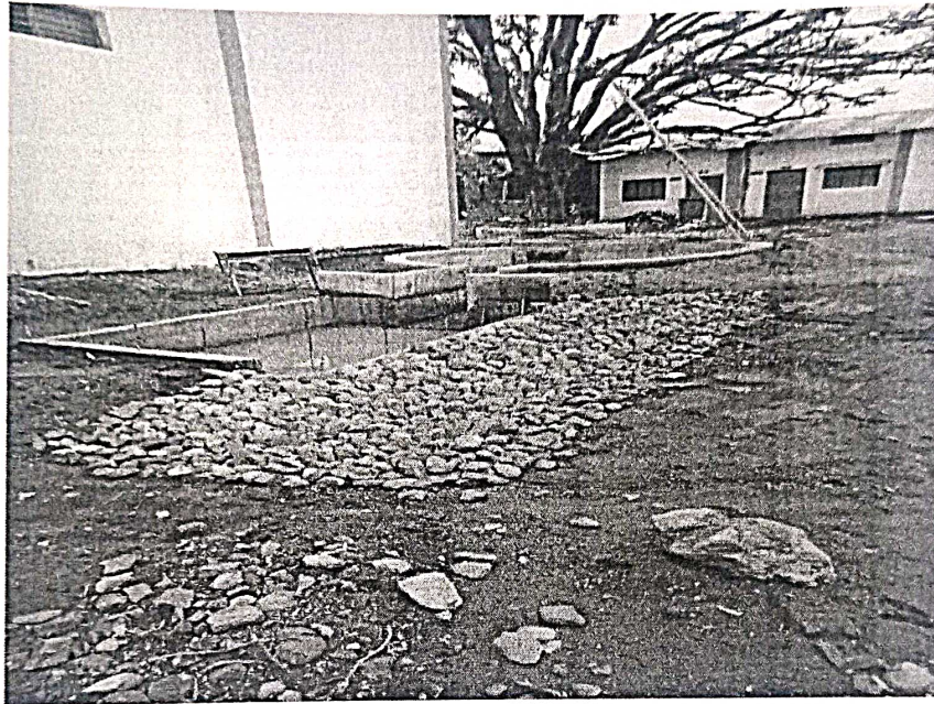
Photograph of Rain Water Harvesting
